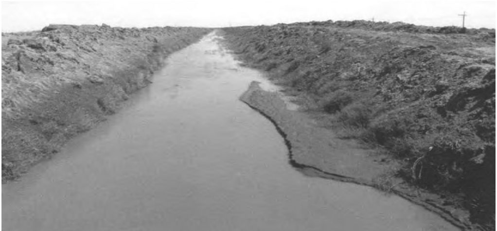
Figure (2) Silt accumulating in a Gezira minor canal, Sudan. As the silt is dug out, the banks grow higher each year
