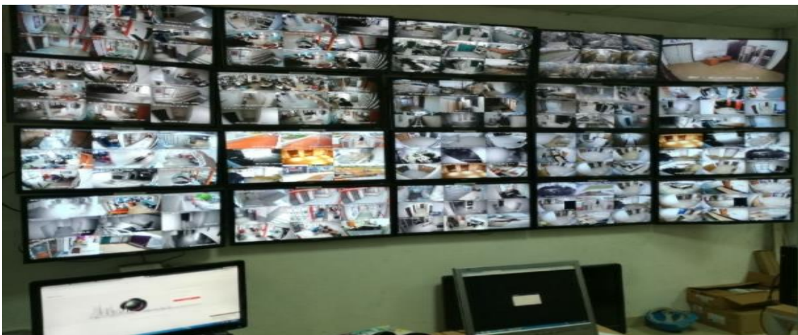
Figure 2. surveillance CCTV system.
